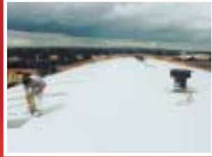
A corrugated metal roof protected from ongoing corrosion with Corro-Tech GP and Uni-Tech UV.
