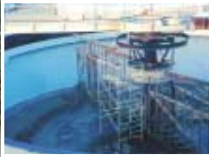
Metal and concrete surfaces of this effluent treatment tank lined with Chemi-Tech EP, a heavy duty corrosion and chemical resistant coating.
